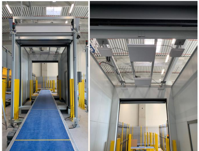
Example: full pallet RFID chamber on conveyor with automatically closing stainless roll-doors reading up to 350 kitchen parts in 7 seconds.
